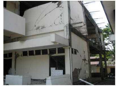
Photo 9 Damage of South-side of the Building
