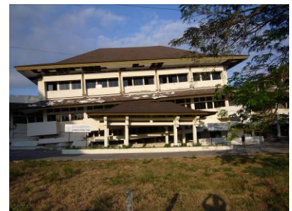
(b) Story-Collapsed Building
