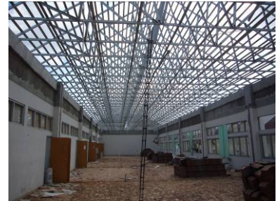
Photo 4 Damage of Roof in UIN
