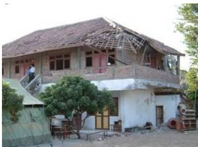
Photo 12 Partial Collapse of Roof
