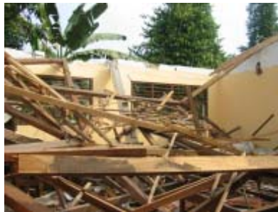
Photo 13 Collapse of Roof Structure
