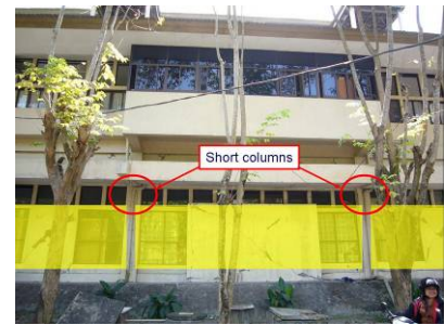
Photo 11 Damage of South Frame of Slight Damaged Building
