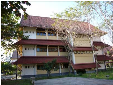
(a) Slight Damaged Building
