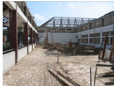
Photo 3 Damage of Roof in UAD
