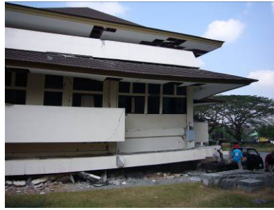
Photo 8 Damage of North-side of the Building
