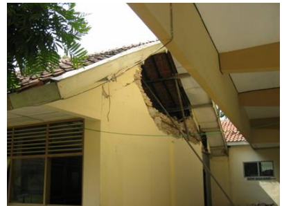
Photo 14 Damage of Unconfined Masonry Wall
