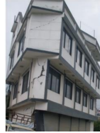
(a) Damage due to torsional effect
