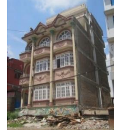
(b) Collapse due to soft story effect
