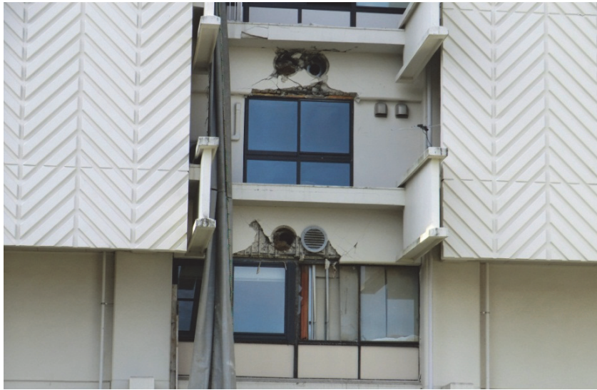
Photo 12 Coupling beams damaged around openings
