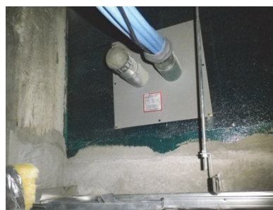
Photo 3 Stuck carbon fiber without anchors
