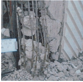
Photo 15 Column of the penthouse after the earthquake
