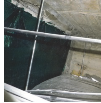
Photo 10 Anchorage failed Floor 7 Frame 11 Beam I-J
