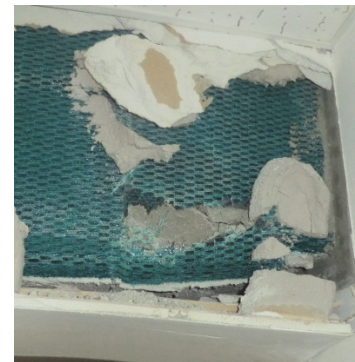
Photo 7 Broken fibers Floor 7 Frame 11 Beam I-J
