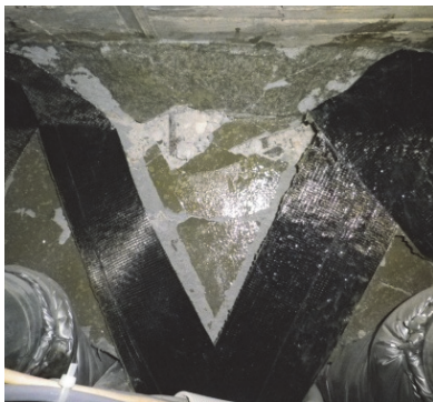
Photo 5 Unstuck tapes Floor 5 Frame 12 Beam I-J
