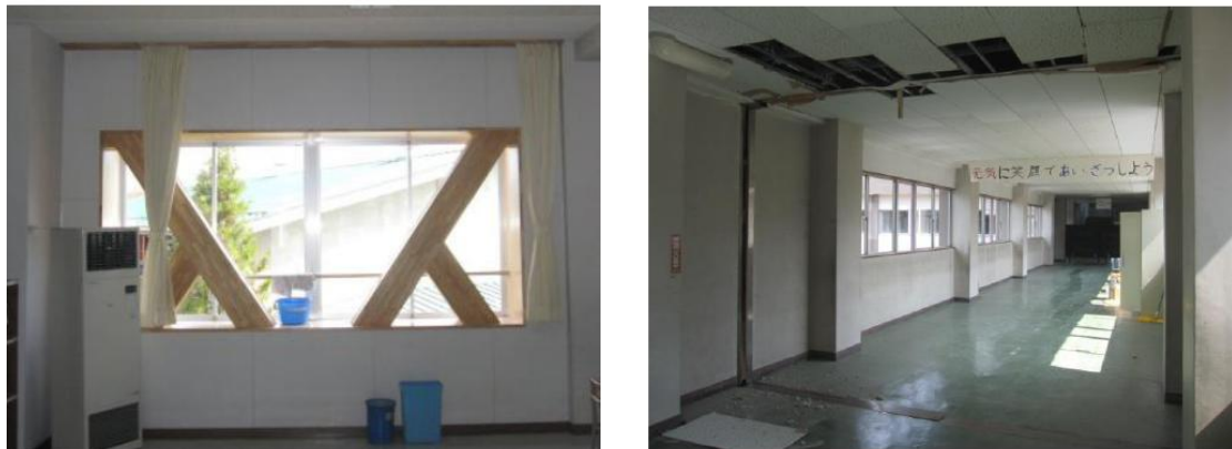
Figure 4-10 Examples of damage of sample building T
