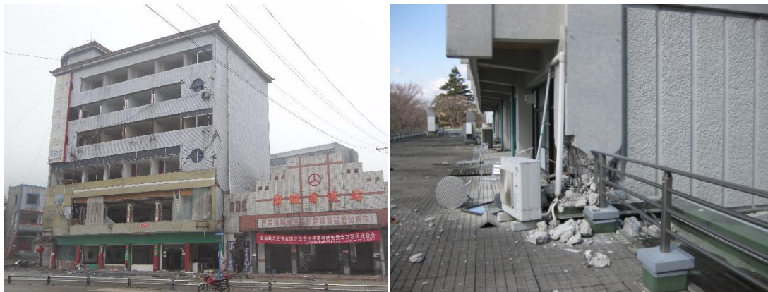
Figure 1-3 Building damaged during 512 and 311 earthquakes
