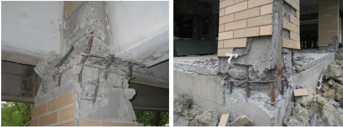
Photo 7 Flexural Compression Failure at the top and Bottom of Columns
