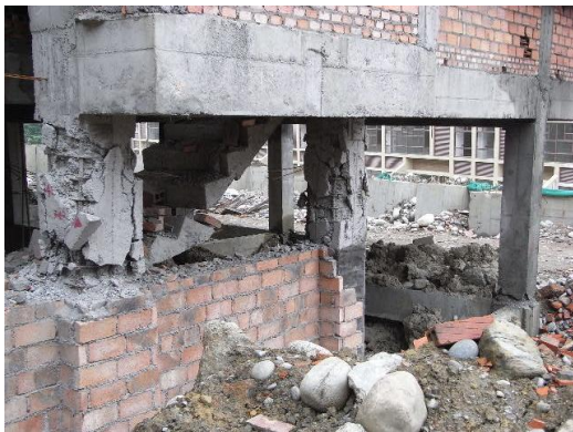
Photo 4. Typical shear failure in RC short columns
