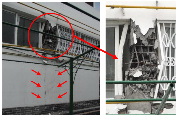
Photo 5. Shear failure in RC column shortened by partial height brick wall
