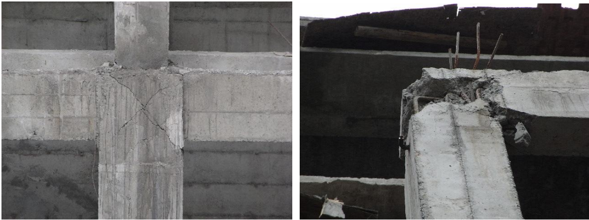
Photo 8 Failure in beam-column joint
